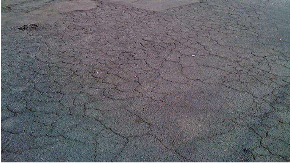
Fig. Alligator Cracking
