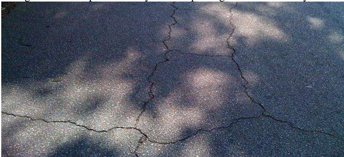
Fig. Block Cracking
