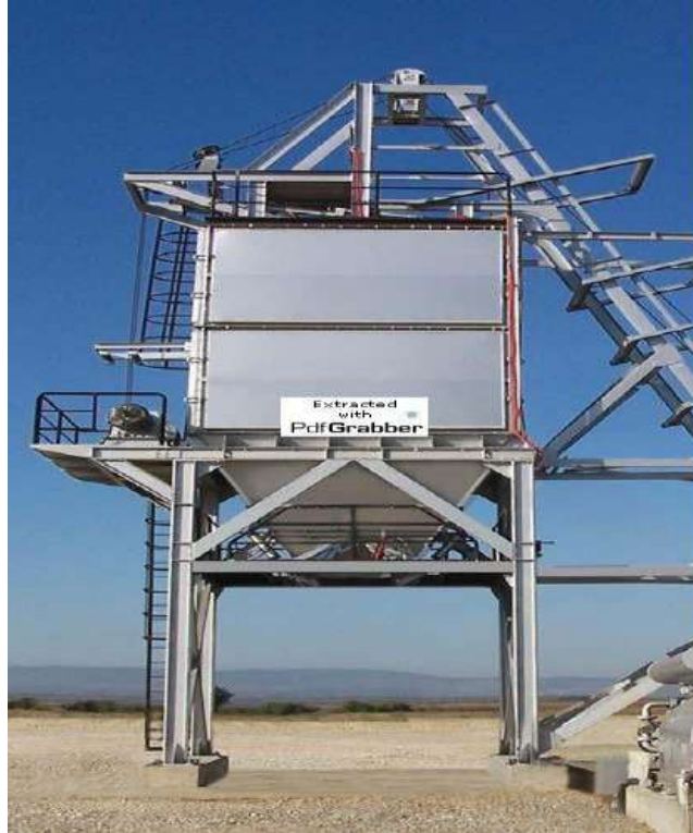
Fig.Hot mix storage silo
