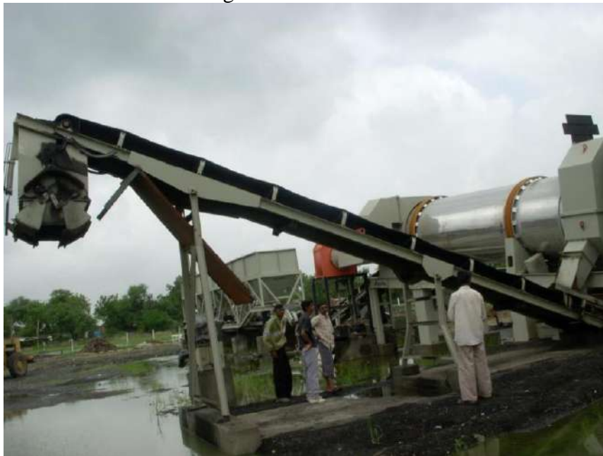
Fig. Load Out Conveyor
