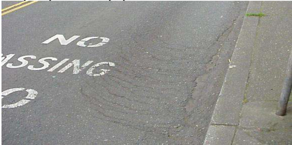
Fig. Slippage Cracks
