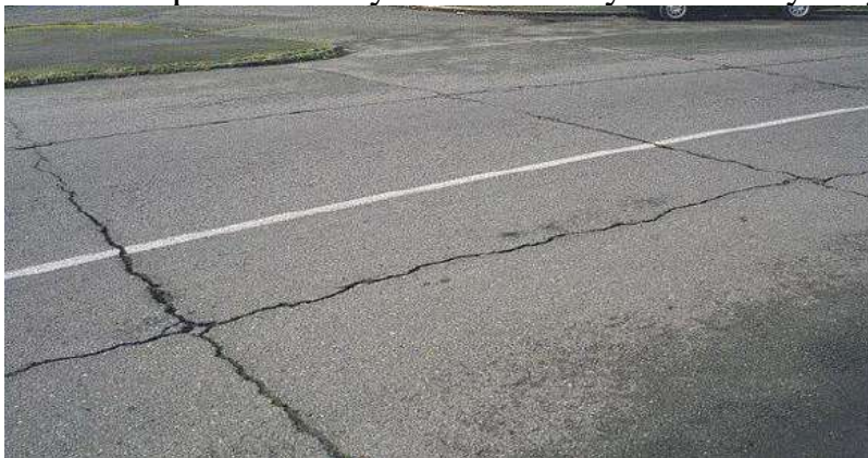
Fig. Joint Reflection Cracks
