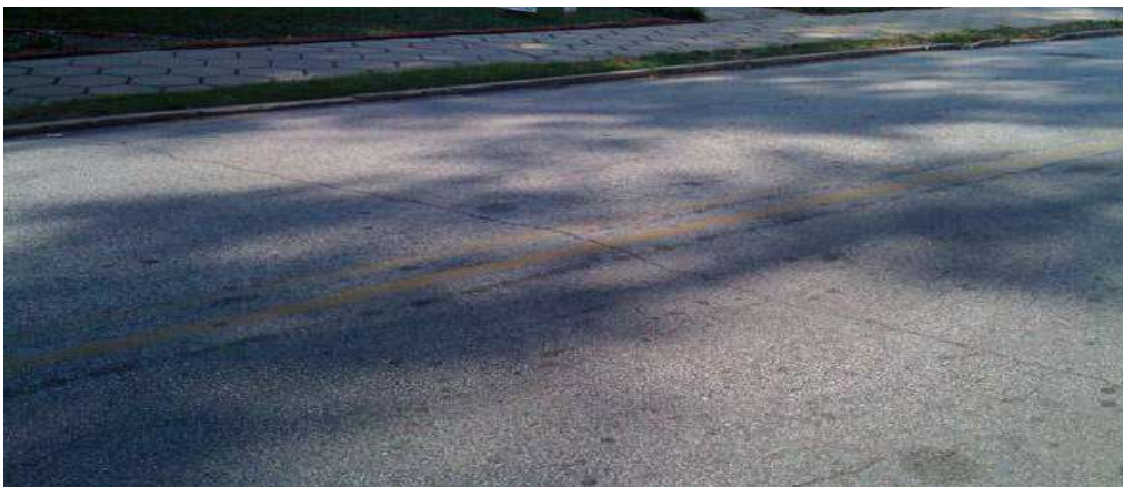
Fig. Transverse Cracking
