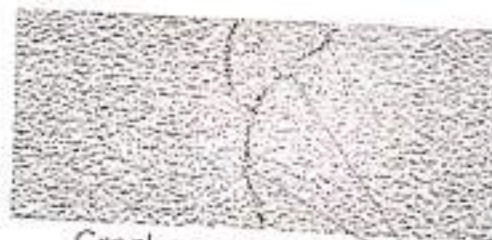
Crack in concrete due to shrinkage
