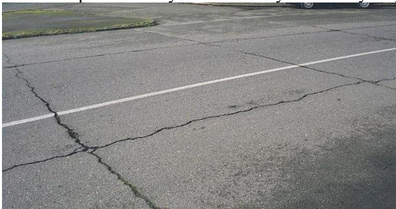
Fig. Joint Reflection Cracks
