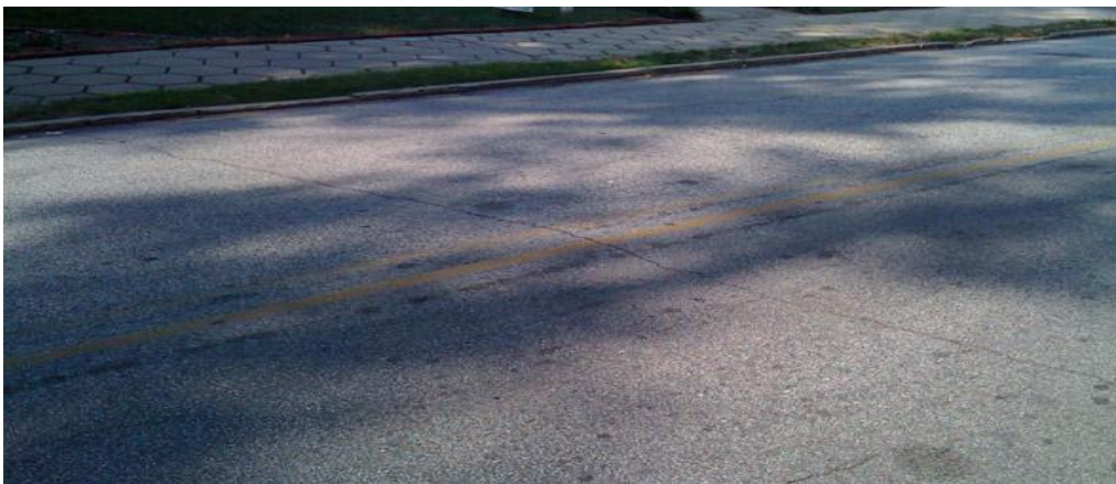
Fig. Transverse Cracking
