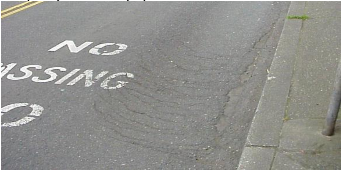
Fig. Slippage Cracks
