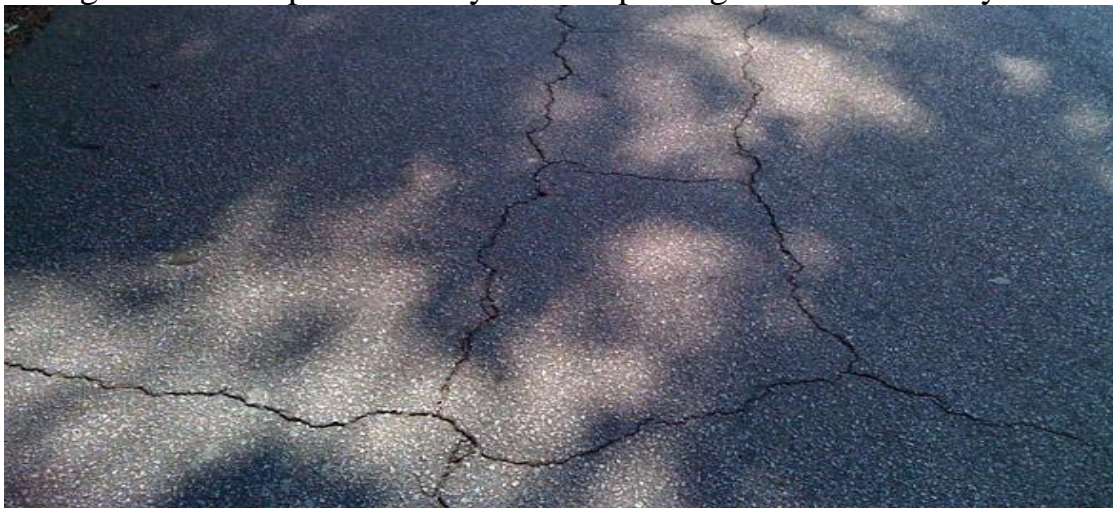
Fig. Block Cracking
